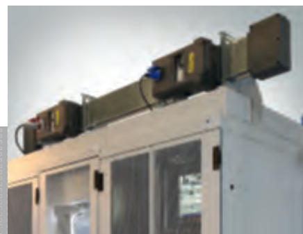
2 Tap-off box over Cold Corridor® → SEE P. 51
