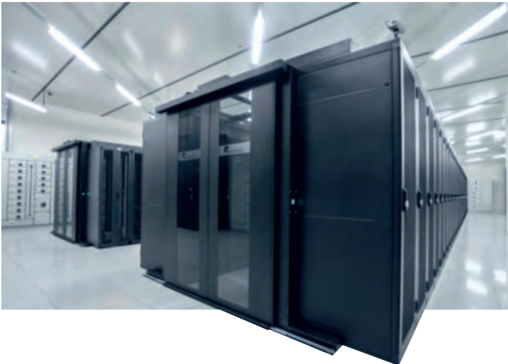
Modular data center
