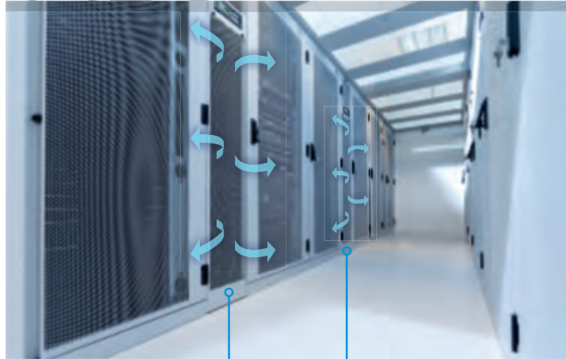
Example of H 2 O in Cold Corridor
