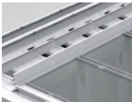
1 Cable management over Cold Corridor® → SEE P. 50
