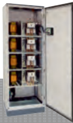
4 Capacitor banks → SEE P. 17
